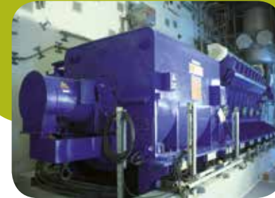
Emergency diesel generators
