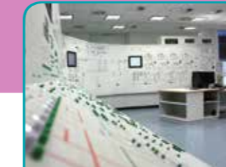
4 Control room with advanced digital I&C systems
